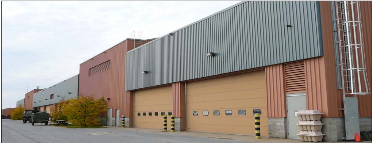
One of the 10 large vehicle maintenance garages that have been retrofitted with grey SolarWall systems at Fort Drum.
