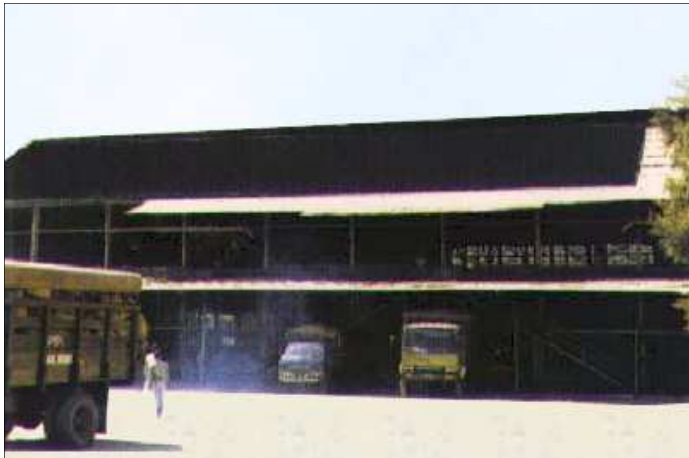
Roof mounted black SolarWall® System
