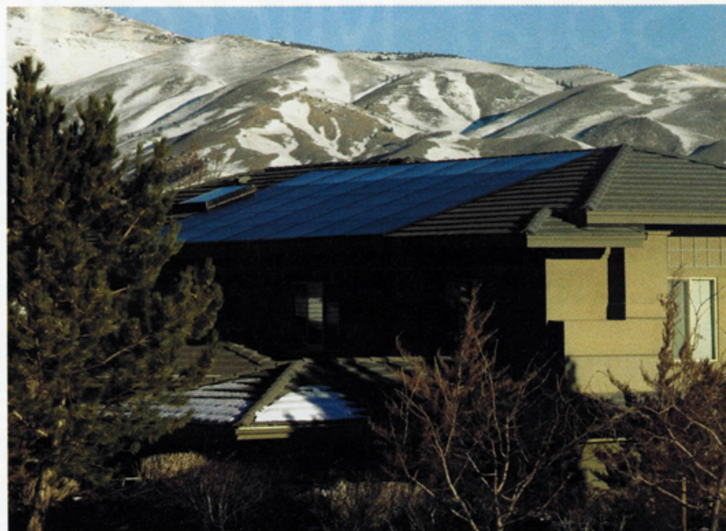
A hybrid photovoltaic/thermal solar installation in Reno, Nev. Photo courtesy of PVT Solar.
