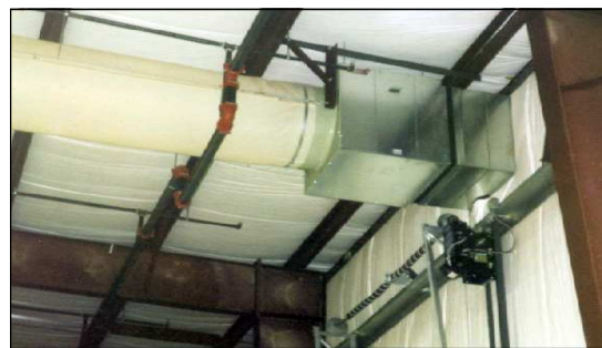
One of three fans and fabric ducting that distribute the solar heated fresh air.
