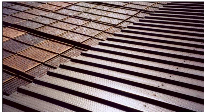
A section of the roof mounted SolarWall® system
