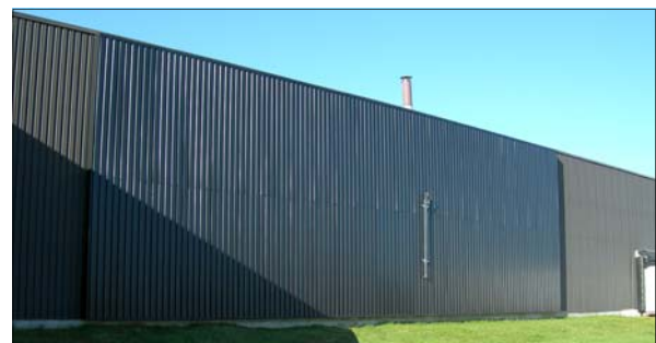
3M Canada's completed SolarWall® system
